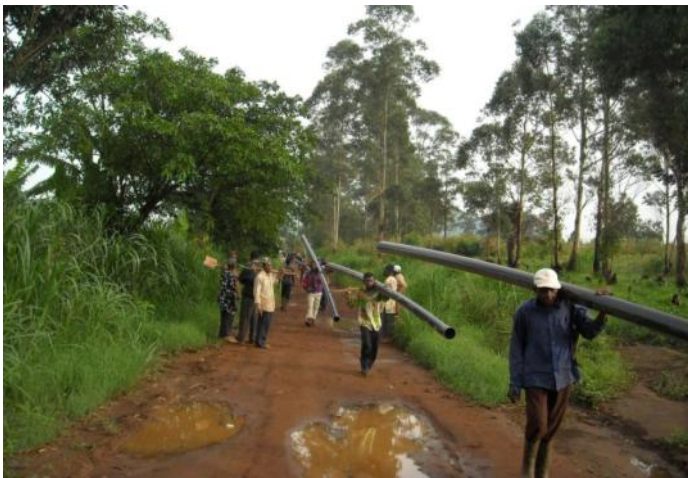
Wum Village residents carry lengths of water pipe to be installed as part of Phase I of the TRF-funded project.
